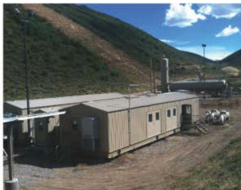
Installation at Encana's site in Piceance Creek has to adapt to the mountainous surroundings of the area.
