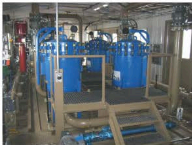
DXP/Quadra's team made sure that the equipment integrated into the packaged pump system.
