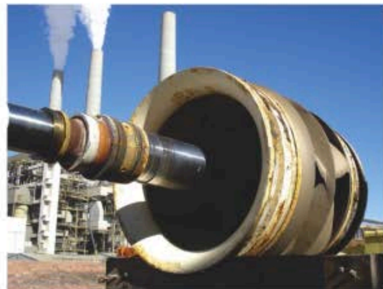
Figure 2. A double suction impeller for one of the cooling tower pumps.
