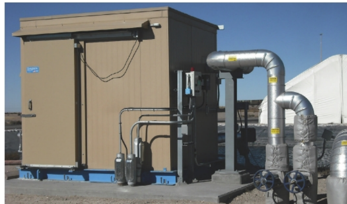
The pumps are enclosed in an 8 x 10 ft glass fibre enclosure. It features ventilation for summer and heat for winter to protect the pumps, piping, valves, lighting and control panel housed within the building. Photo: Quadna.
