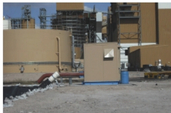
Pump house enclosure unit that processes the plant's effluent water. Photo: Quadna.
