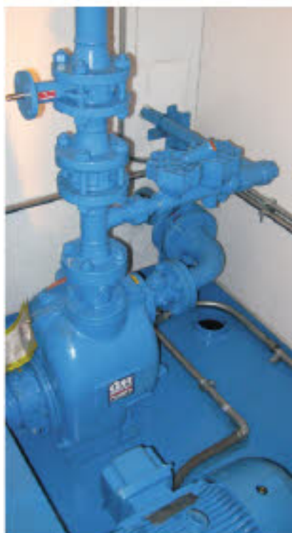
The pump house enclosure unit. Photo courtesy Quadna.
